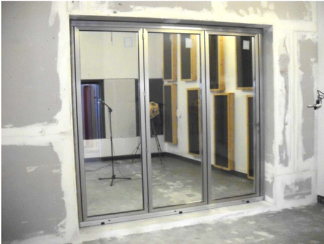
Fig. 1: View Transmission Room
